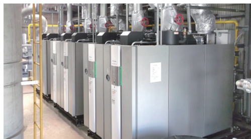
High-efficiency, energy-saving gas boiler facilities (Kashima Plant-West)
