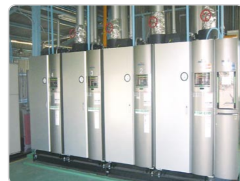
Upgraded boilers at the Akashi factory
